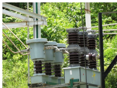
Kasipatnam Substation Visit in 12 th September 2013
