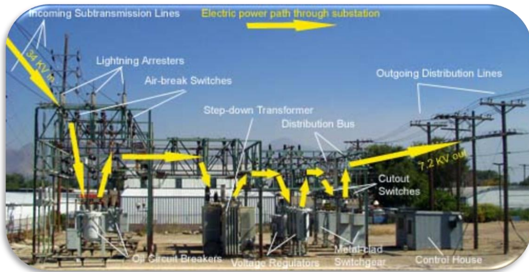
Figure 4.1 A Typical Substation
